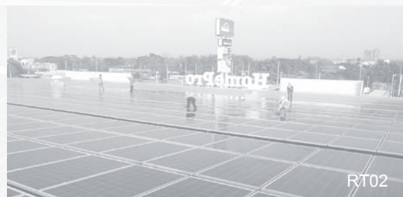
Location HMPRO Muang District, Phrae Selling Capacity 1 MW COD 3 Feb 2015
