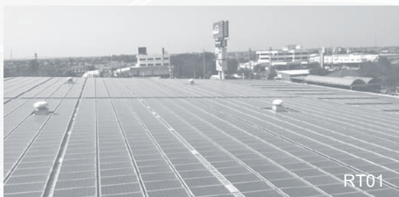
Location HMPRO, Muang District, Lopburi Selling Capacity 1 MW COD 4 Sept 2014
