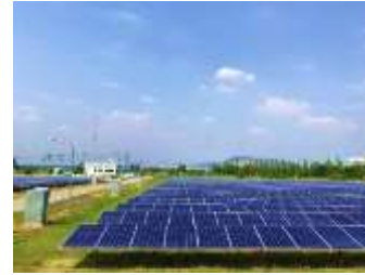
SSE1-PV09 (8MW) COD APR 2014
