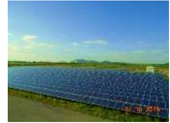
SSE1-PV06 (8MW) COD JUN 2014
