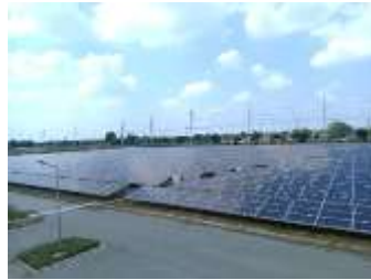
SSE1-PV02 (8MW) COD JUL 2013
