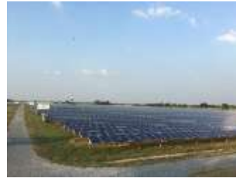
SSE1-PV03 (8MW) COD OCT 2013
