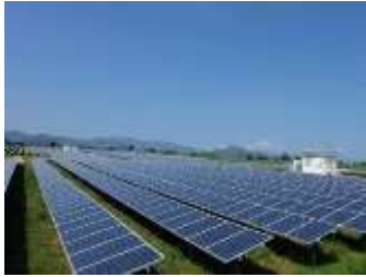
SSE1-PV01 (8MW) COD SEP 2013
