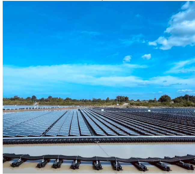
Floating Solar PV
