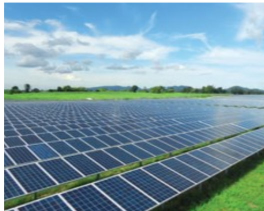
Solar PV Farm
