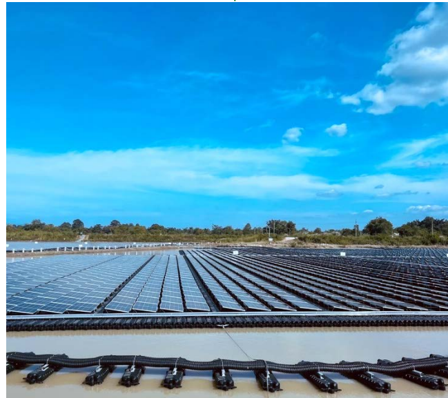
Floating Solar PV
