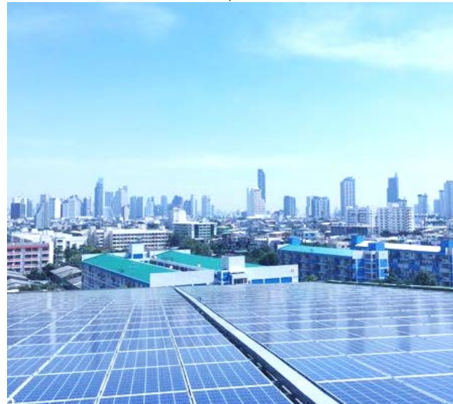
Solar PV Rooftops
