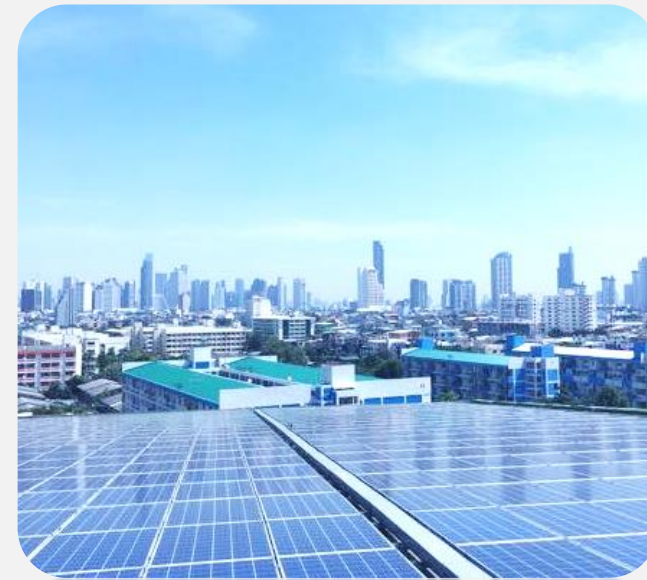
Solar PV Rooftops 14 MWac
